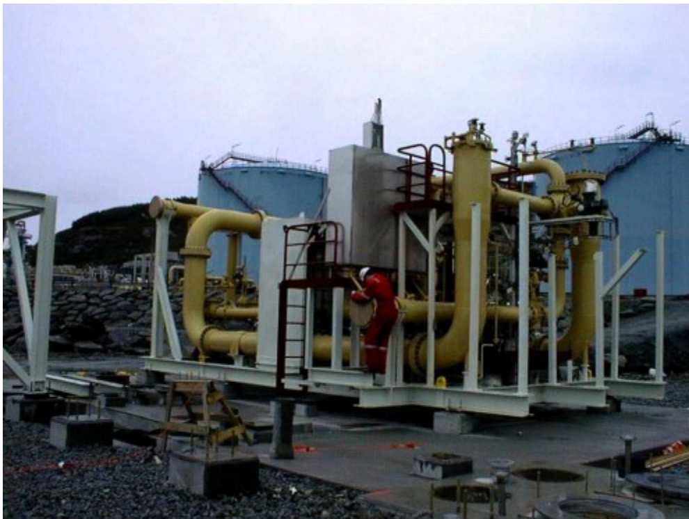
Figure 4 Ü Metering Station
